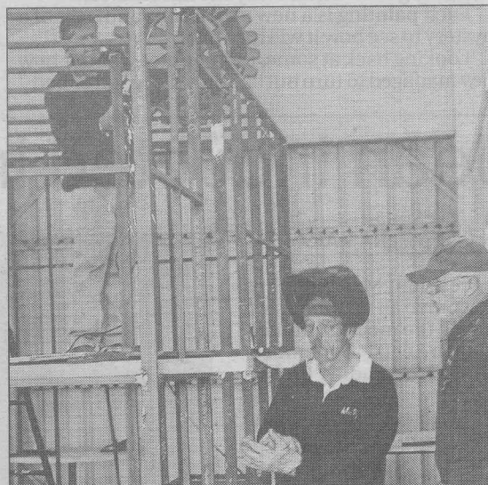
Soto Stuppos (rear), Alistair Stevenson and Brian Moody busy constructing the new catering van.
